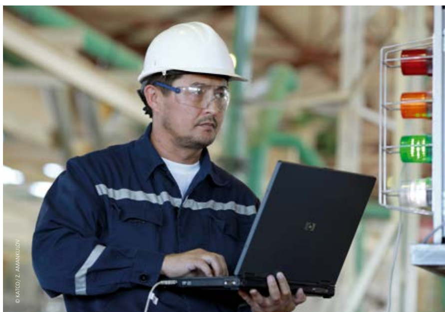
Control of radon measurement device at the plant
